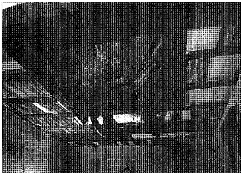
PHOTO NO.5: Corroded steel of abandoned aggregate chute.
