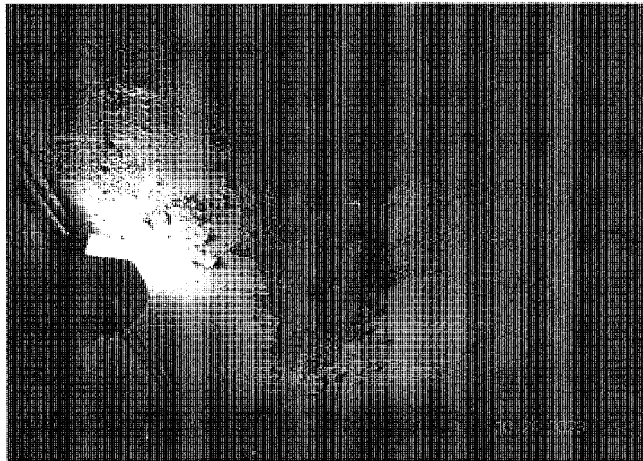
PHOTO NO.9: Crack with active water infiltration and rust staining on underside of roof slab.
