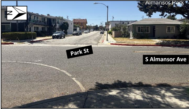
View of existing ADA-ramp on the north-west corner of Park Street and South Almansor Avenue.
