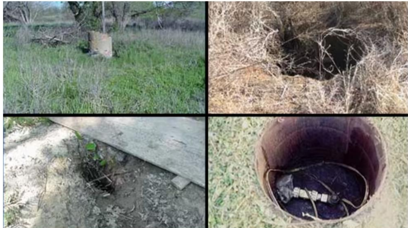
Top Left: Large diameter/hand dug abandoned well, Top Right: Abandoned well open hole, Bottom Left: Abandoned well covered with plywood, Bottom Right: Abandoned well with casing and pump. (Texas Department of Licensing and Regulation)
