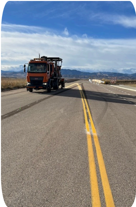
Colorado Barricade removed the existing double yellow center line on County Road 10E to allow for the rerouting of the drive lanes due to the installation of the delineators on the bridge.
