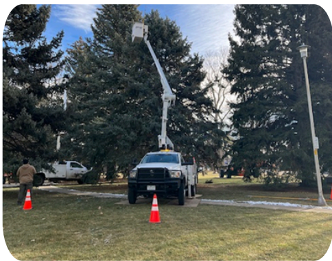
Forestry and Open Space staff worked with the contractor putting lights up in Fickel Park.
