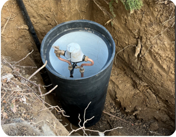
A new water meter and curb stop valve were installed at 353 Michigan Avenue to improve service reliability.
