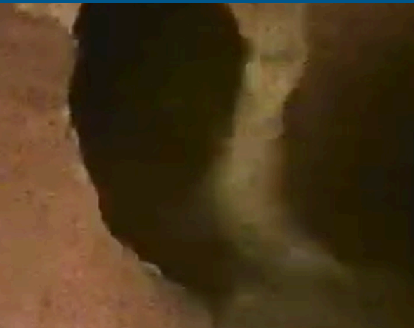
Hole in Sidewall of Pipe
