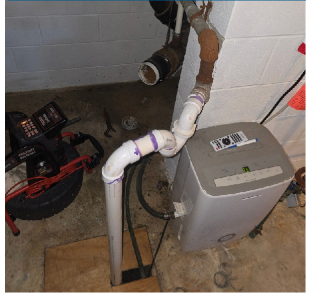
Illicit Sump Pump
