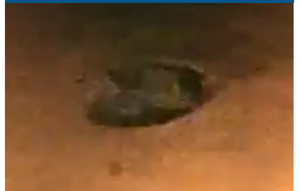
Rock Punched Hole in Pipe
