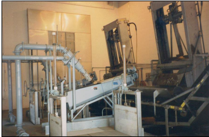
Bar Screens & Grit Removal
