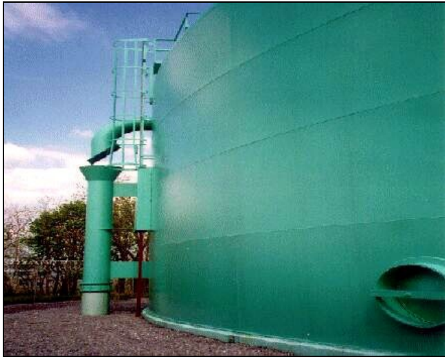
Plane 9 Water Storage Tank
