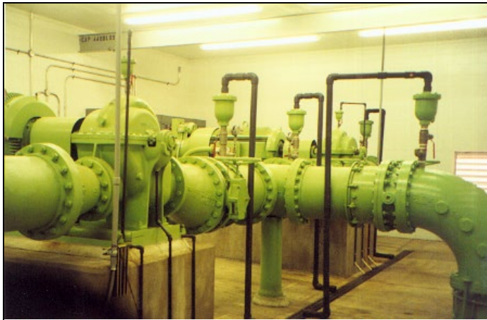
Pumping Station Interiors
