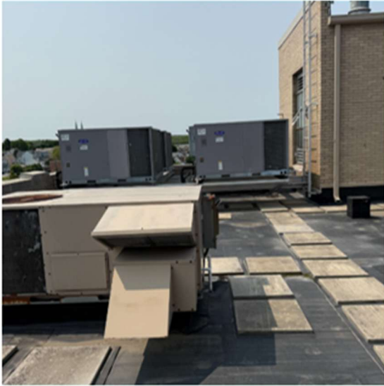
Roof Top-HVAC Unit
