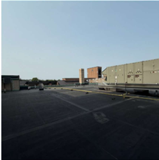
Roof Top-HVAC Unit
