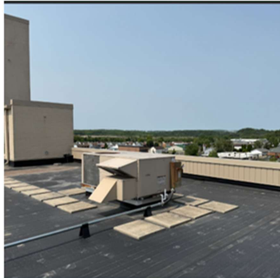
Roof Top-HVAC Unit
