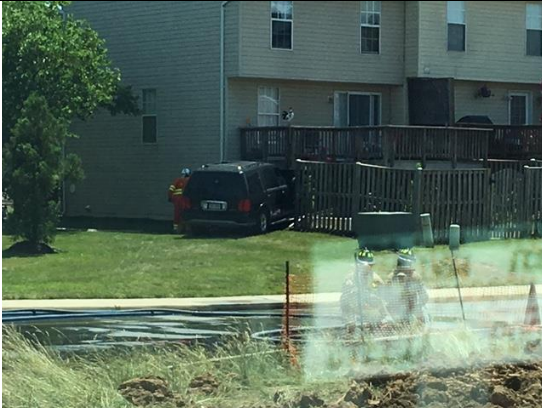
Vehicle into deck and damaged gas meter.
