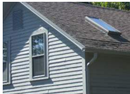
A standard aluminum ogee gutter and downspout blend with the building by matching the paint color.
