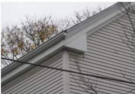
The ubiquitous “pork-chop” eave return applies a triangular box at the intersection of the eave and rake.
