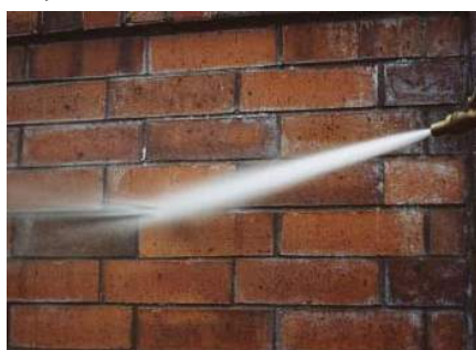
Sandblasting is harsh and can erode the brick and mortar.
