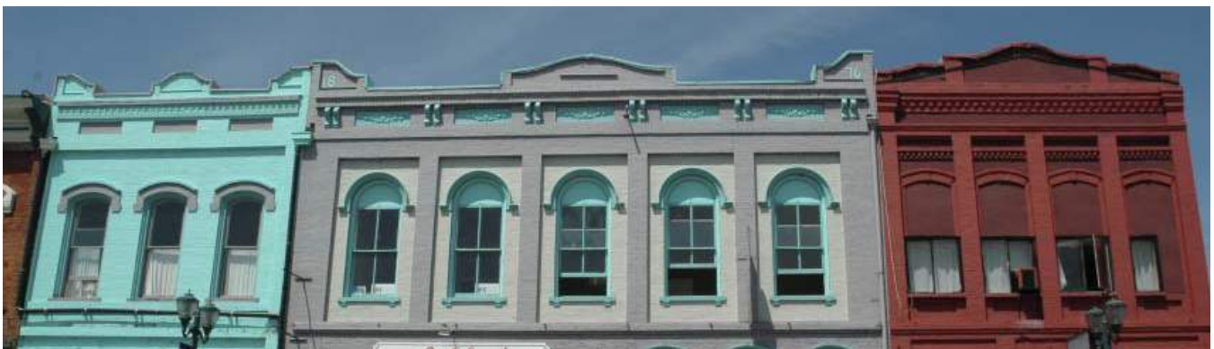
Parapets give expression to the top of a building, articulated and detailed in keeping with the rest of the facade.
