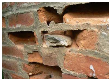
Cement mortar is incompatible and may cause historic brick to erode.
