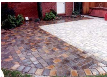
Sealant applied to existing brick or stone will discolor the masonry.
