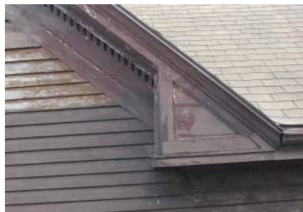
This historic eave return was later enclosed with flat trim.
