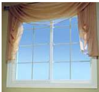
Tight-mulled windows have only a narrow vertical bar between units. This mull should be wide enough to separate two distinct window units.
