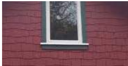
Jagged edges caused by alternating shingle exposures. Traditional shingle siding is aligned in horizontal courses.
