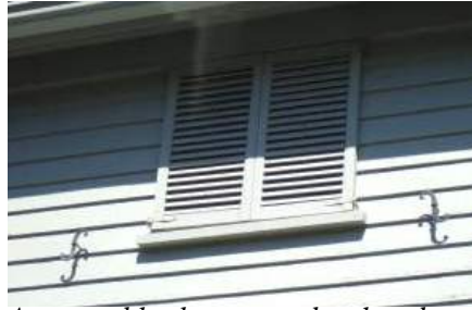
An operable shutter can be closed when the room is not in use.
