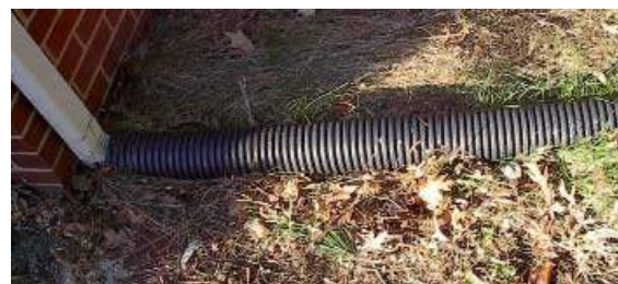
Extension hoses are unsightly additions and call attention to the poorly designed gutter system.
