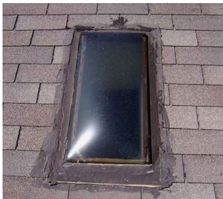
Skylights with a high profile or strong color contrast with the roof stand out.
