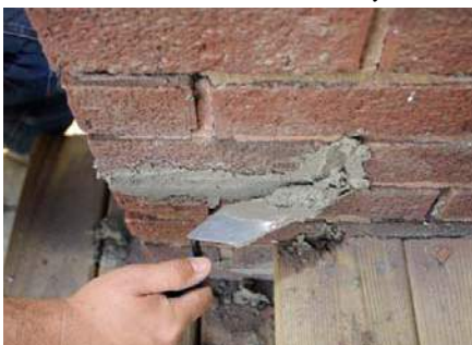
Sloppy re-pointing may leave excessive mortar on the face of the brick.
