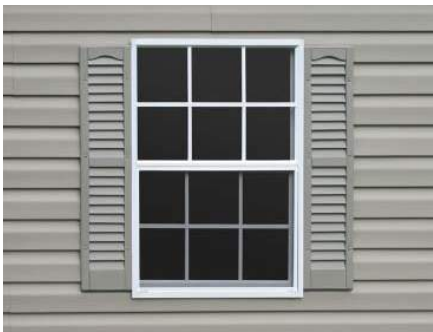
Inappropriately sized or poorly located shutters would not cover the window if they could be closed.
