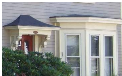
Metal roofing is common on low pitches over porticoes, porches and bays.
