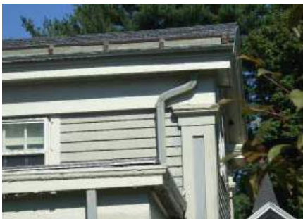
Built-in gutters use the inside of the eaves to channel water flow.
