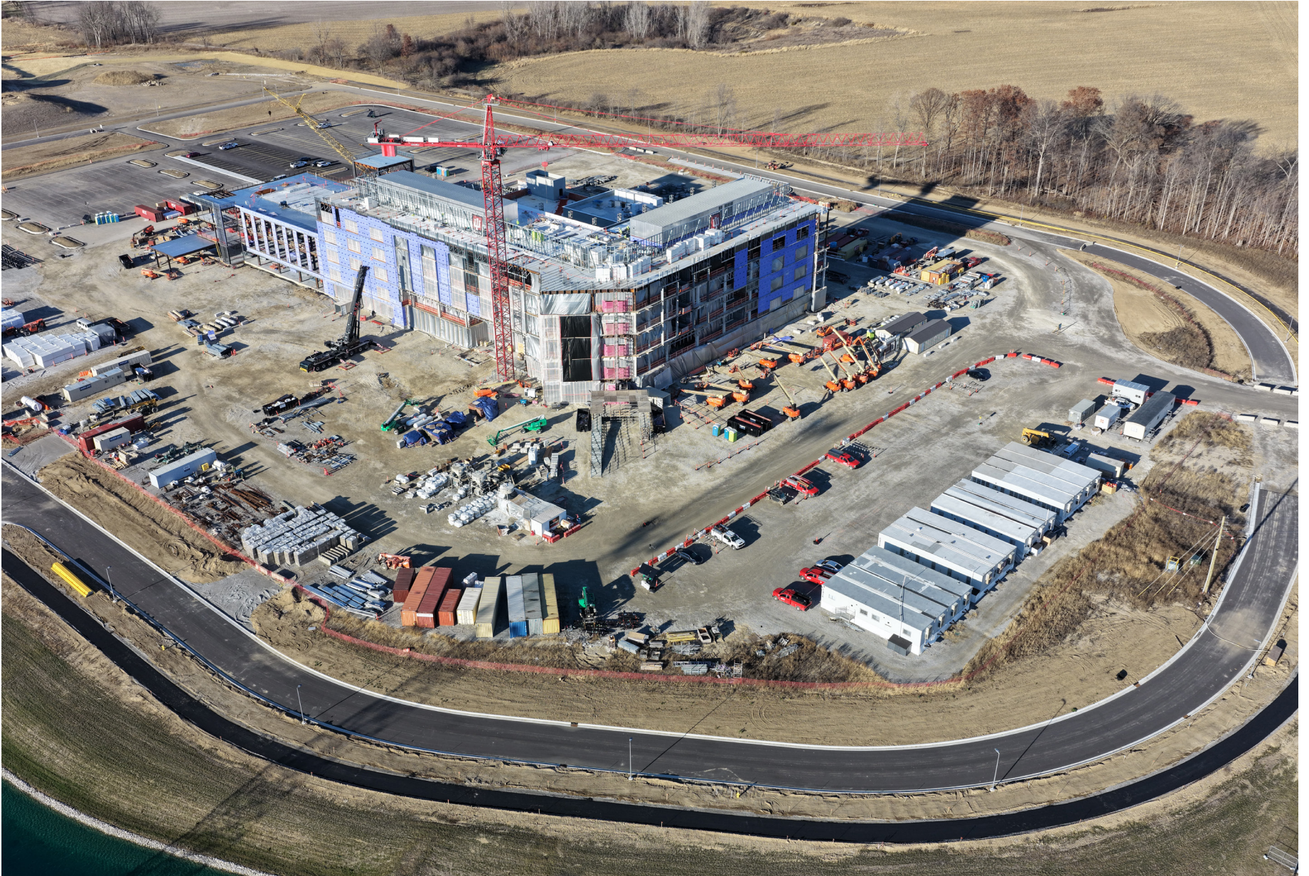
A topping out ceremony was held in July 2025 on IU Health's new hospital in the Prairie Centre Economic Development Area/Allocation Area.
