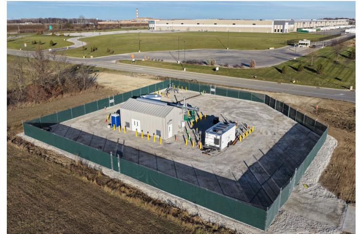
The completed NIPSCO natural gas regulator station in Stonebridge Business Park
